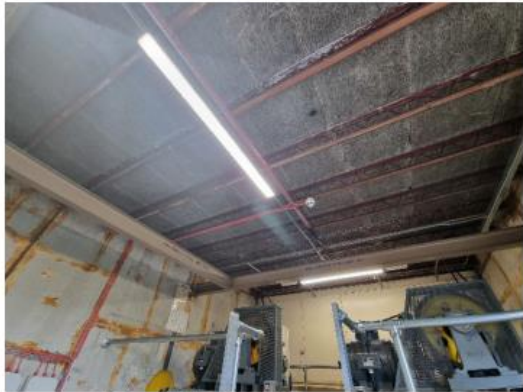
New PIR lighting system
